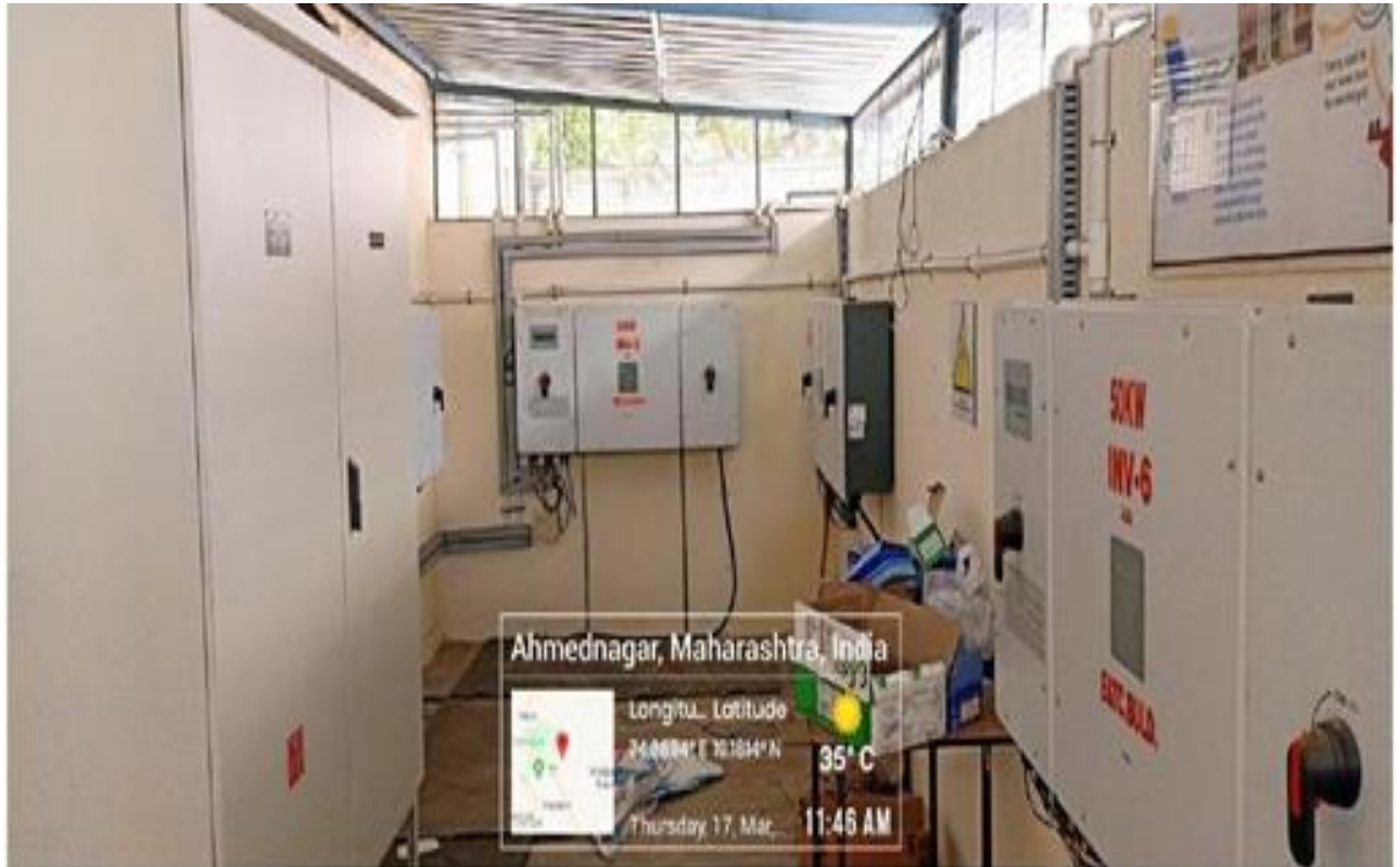
Solar Energy system and wheeling to the Grid
